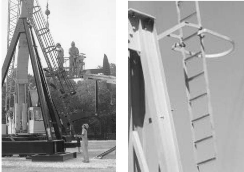
Figure 28: On left, ladder prior to attachment to Samson Post. On right, ladder with support loop installed in area of Center Bearing.
