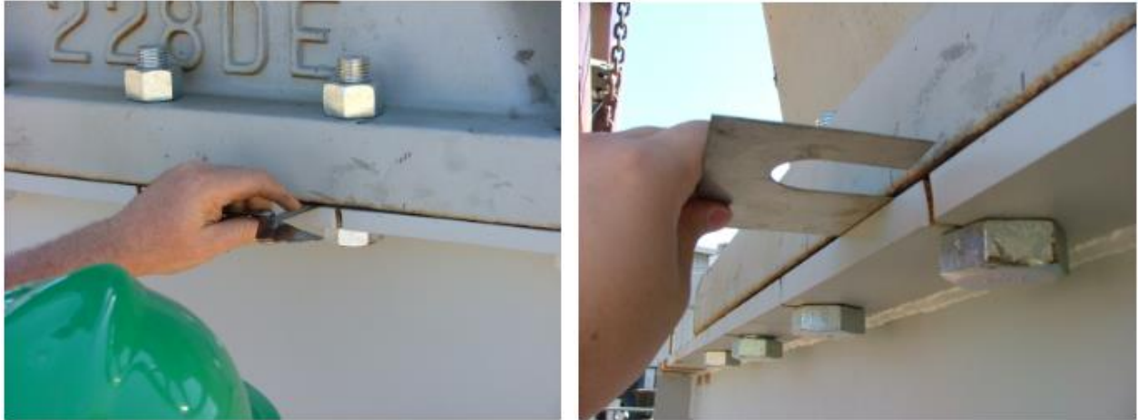
Figure 20: On left, verification of gap between reducer and sub-base. On right, installing steel horseshoe-shaped shim.
