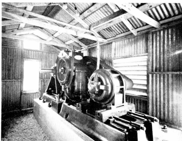
Interior View of Sun Oil Company, Walker No. 1, showing regular electric motor drive for Lufkin 5 1/2" Unit, mounted upon Lufkin Universal base.
