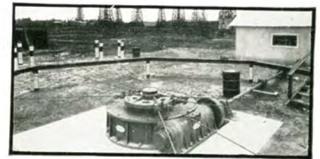
Typical Lufkin Central Power Installation
