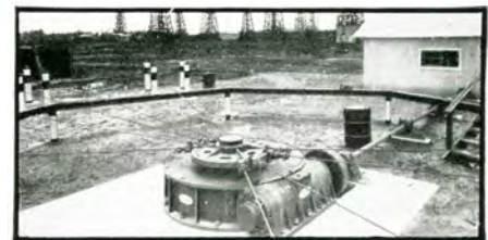
Typical Lufkin Central Power Installation
